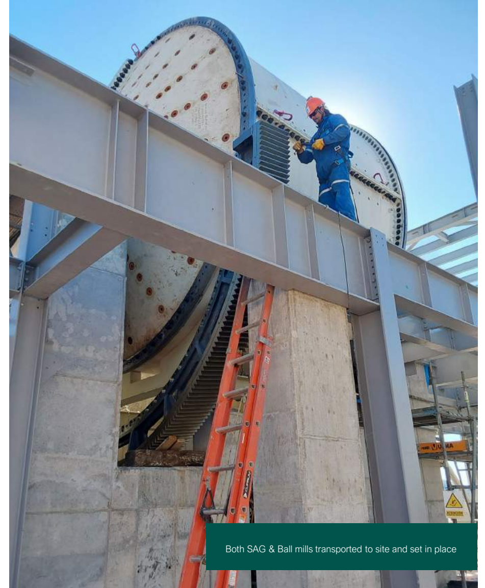
Concrete work for the floor area and steel installation underway at the flotation and thickener locations
